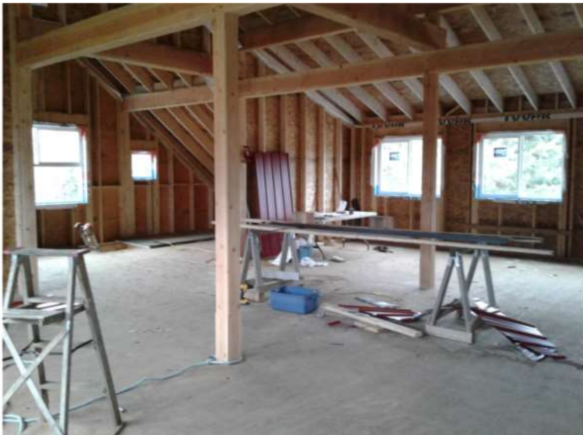
Figure 3: Building Under Construction; Dwelling Proposed to be Located on Second Floor (Photographs taken February 25, 2020)
